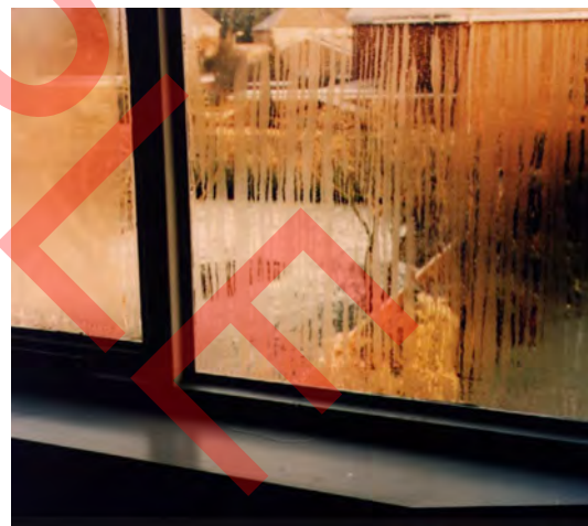
Condensation on inner face of double-glazed windows. Note ponding on sill
