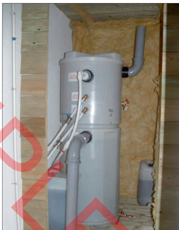
Figure 1: Brac 51 greywater harvesting system filters water from baths, showers and laundry to be reused for flushing WCs and watering the garden
