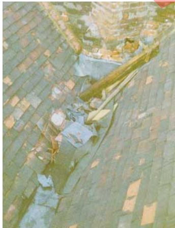
Old roof with frost-damaged tiles needing extensive repair or re-covering
