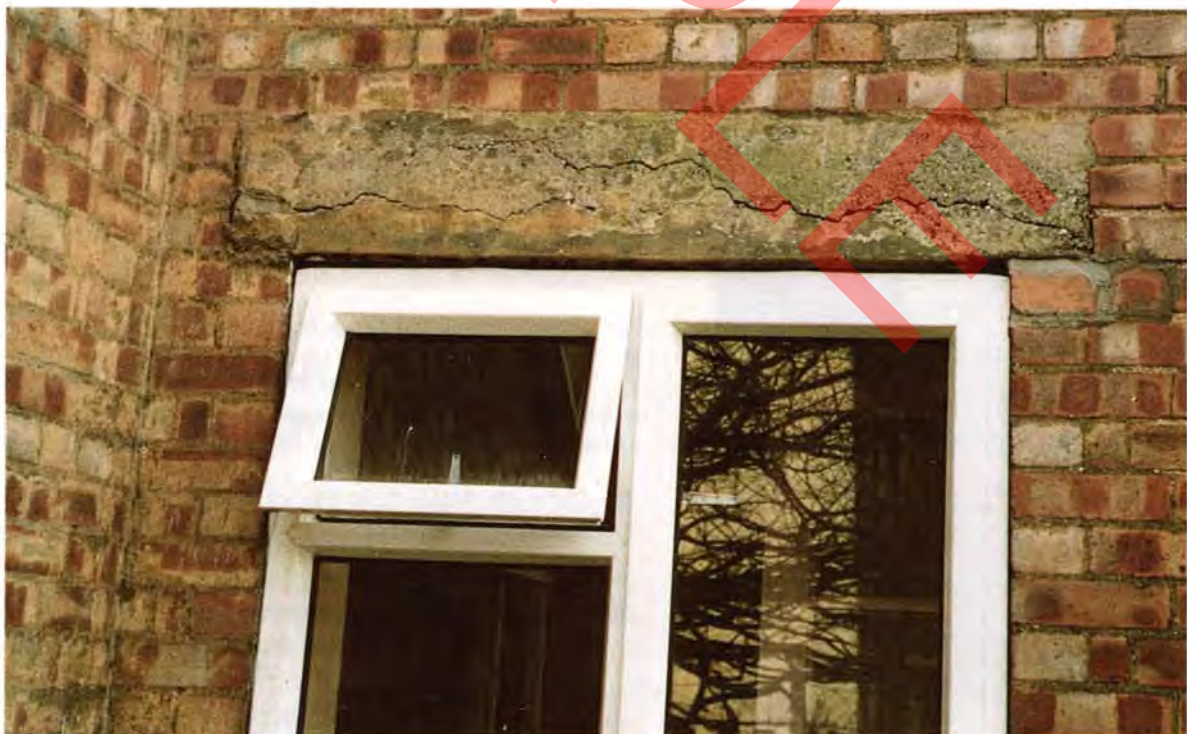
Can this lintel be repaired, or should it be replaced?
