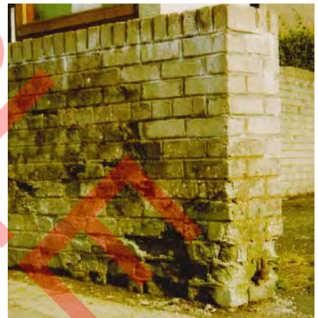
Further frost damage to 28-year-old concrete brick wall following repairs to the frost-damaged coping and end, about 10 years after being built
