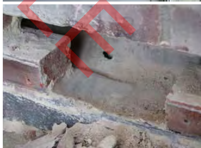
Figure 1: Damage to a ground-floor flat caused by rain penetrating the inner leaf of a cavity wall via a torn and debris-filled cavity tray to a cavity wall of a flat upstairs
