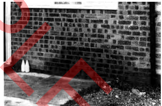
Typical rising damp stain on an external wall. In this case, the dpc was bridged by the paving
