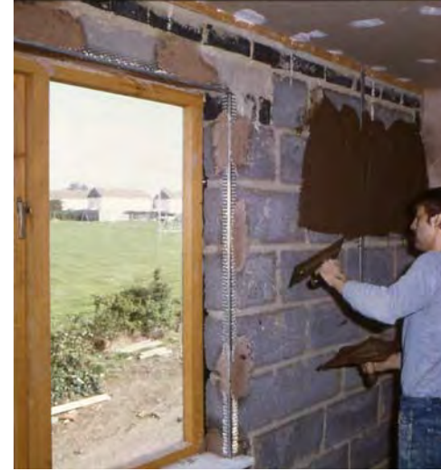
Figure 1 Application of the base coat of render. Note the beads in situ around the window opening
