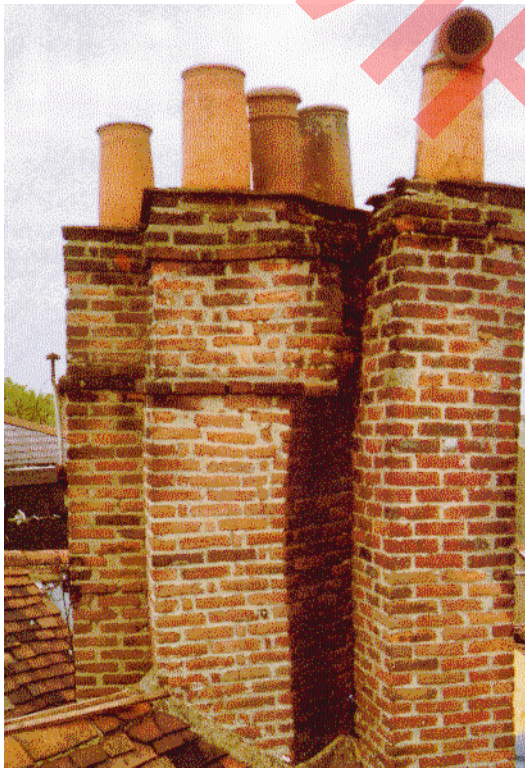
Condensation leading to sulfate attack has caused twisting and leaning of the stacks
