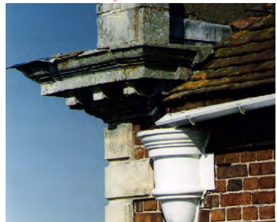
Many houses have defective gutter installations, which can soon lead to dampness problems
