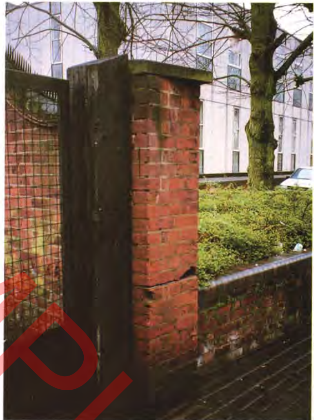
Cracks on or near piers will require urgent attention
