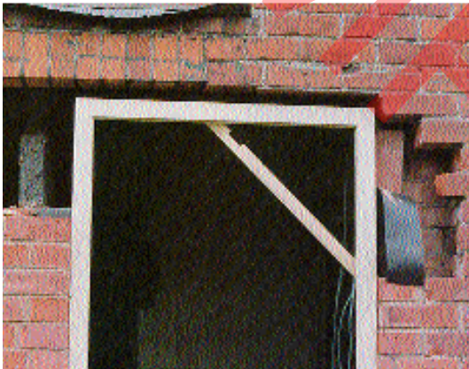
This new door is being fitted without any temporary support to the brickwork above — it could be an expensive mistake
