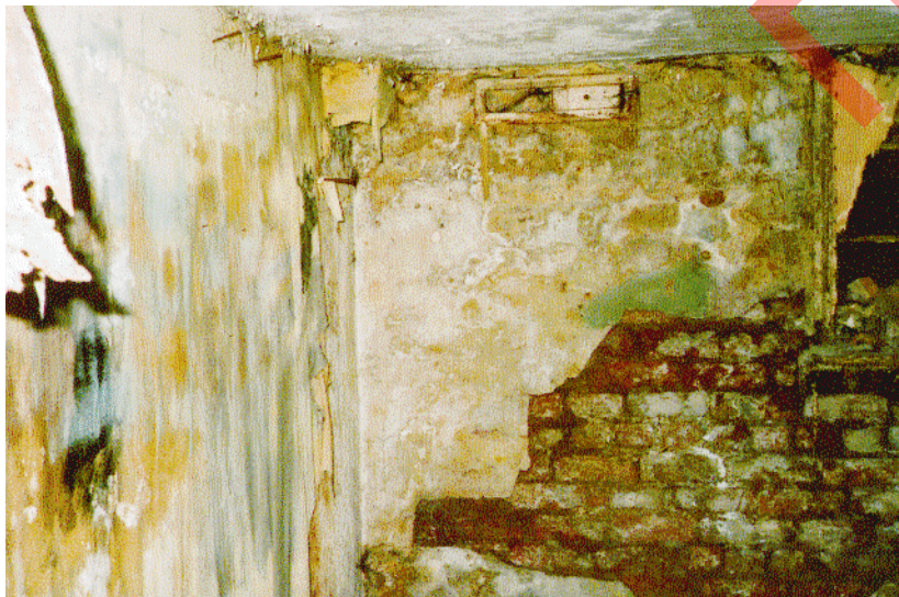
Salts from dampness in the structure is one of the problems to be faced in converting a basement to living space
