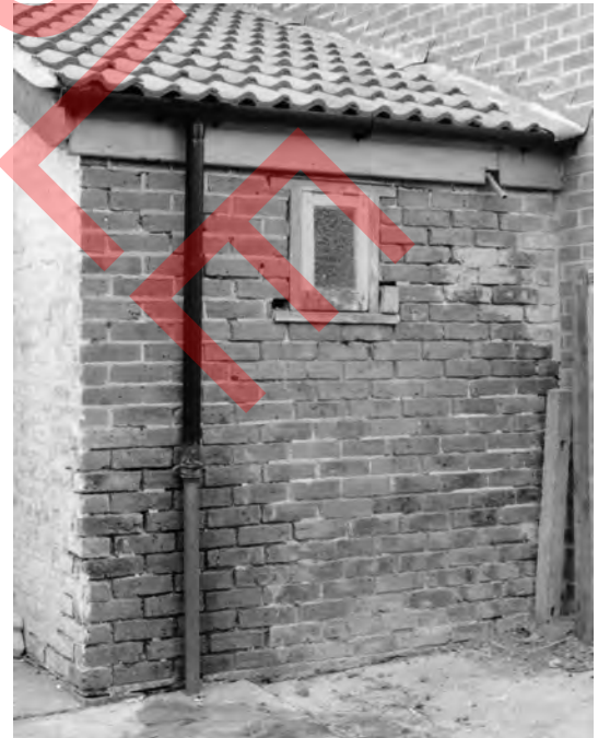
Mortar joints around downpipe have eroded and repointing has been inadequate
