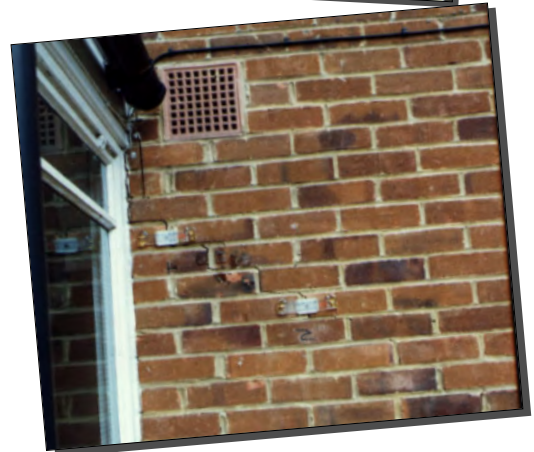
In top pictures, plaster removed to show cracking
