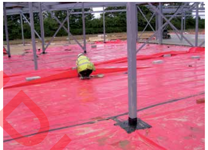
Figure 1: General view of a radon barrier laid over fill and sealed to columns
