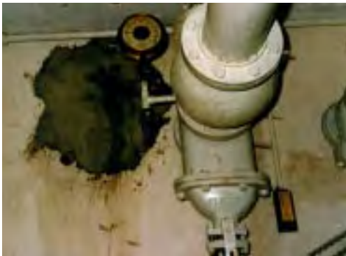
Figure 8 Services passing through the basement wall must be properly waterproofed otherwise leakage (as seen in the photo) may occur
