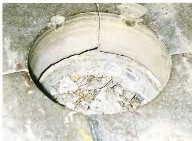
Figure 1 Core through cracked screed. This core was taken at the intersection of four shrinkage cracks and shows clearly that the screed has lipped and curled.
