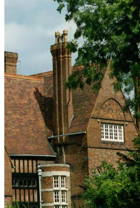
Figure 1 Every tile in this roof should have been twice nailed
