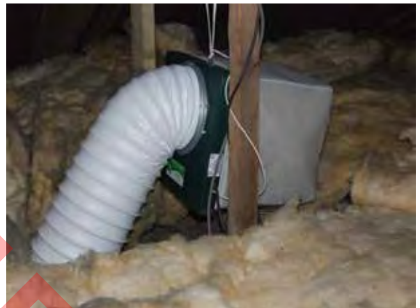
Figure 1: Roof-located positive ventilation system
