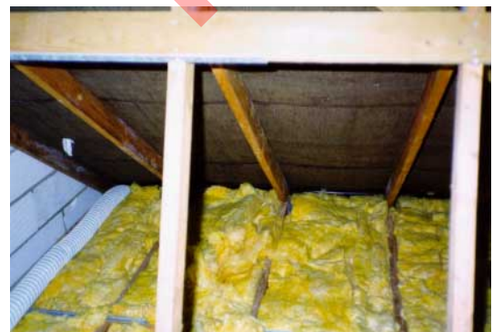
Insulation packed into the eaves has blocked ventilation paths. When the insulation quilt was lifted it was saturated with water condensate
