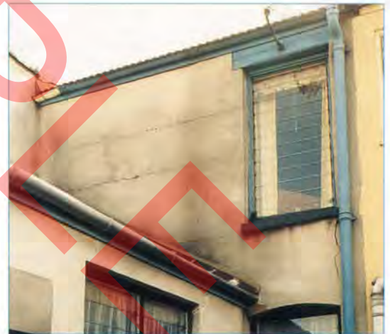
A rendered wall in poor condition. The rendering is discoloured and cracked and has become detached.
