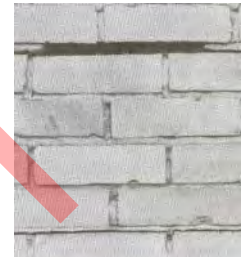
Spalling of thickened joints in fair-faced brickwork
