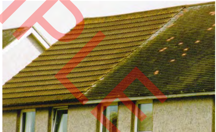
Different strategies for 30-year-old houses. Left, roof re-covered with concrete tiles. Right, frost-damaged clay tiles replaced
