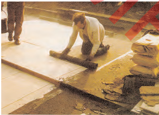
Laying a vapour control layer in hot bitumen over a chipboard deck — the first stage in a warm-deck roof
