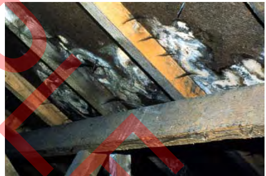
Condensation in the roof space can lead to mould growth and rot in the timbers
