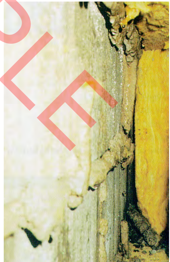
Mortar extrusions into a fully filled cavity can lead to rain crossing to the inner leaf
