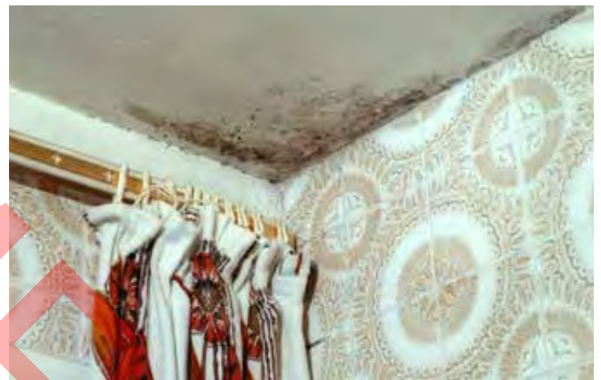
Figure 1: Typical example of mould caused by condensation
