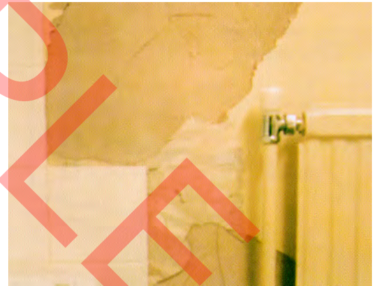
Figure 1 Problems continue to arise due to both short-term and long-term failure of the bond of tiling to its background or adhesive
