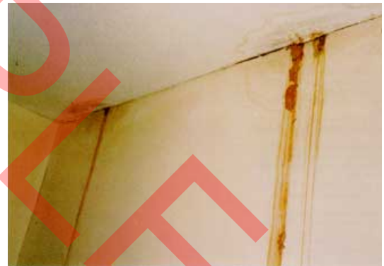
The cost of damage caused by water from a burst pipe is often out of all proportion to the cost of protection from freezing
