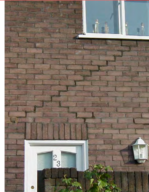
Retro-installation of bed joint reinforcement could be applied to these shrinkage cracks and the dropped flat arch
