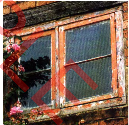
Windows in this kind of neglected condition can be brought back to life provided no serious decay has occurred
