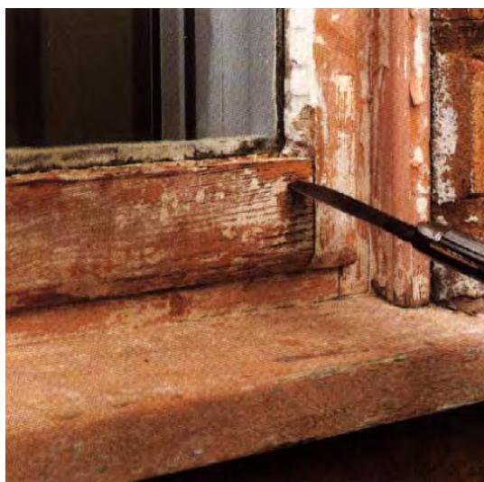
Early stages of decay in a softwood window
