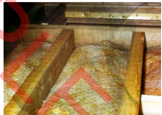
Typical ceiling insulation in a cold pitched roof
