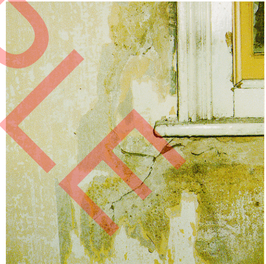
If plaster is damaged by dampness or cracking, it is vital to find out the cause before replastering
