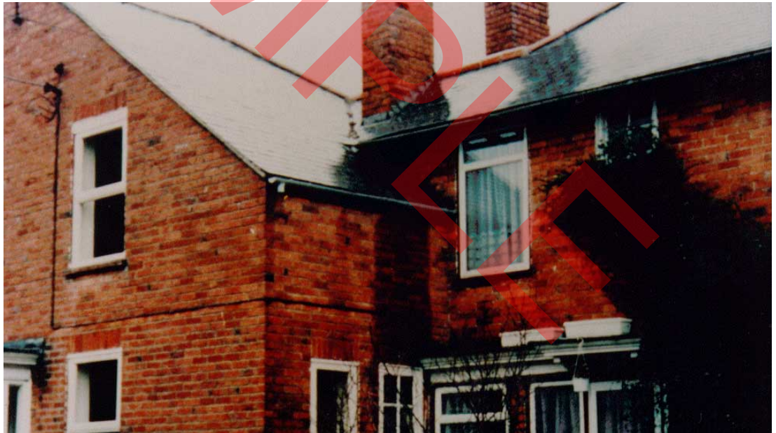
Several defects in the roof drainage are contributing to this damp wall — the downpipe is missing, the gutter slopes the wrong way and is probably undersized for the large area of roof draining into it
