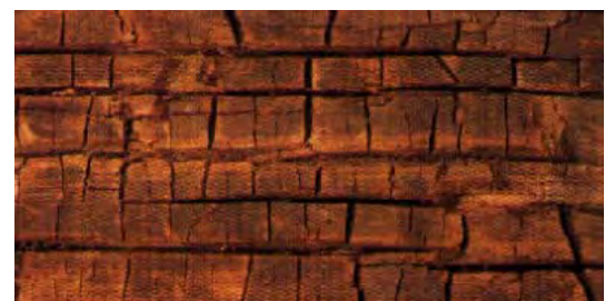
Dry rot damage, showing cube-like cracking
