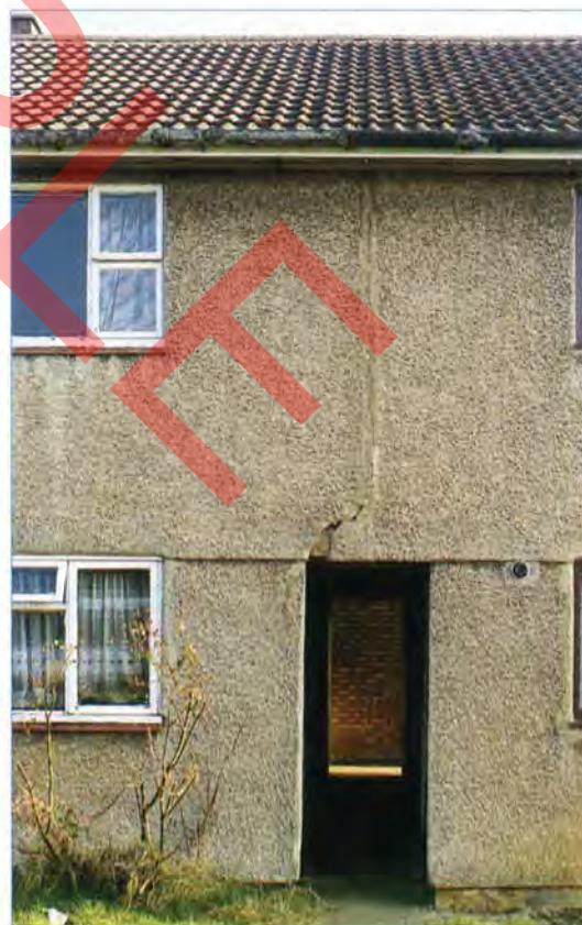
Vertical cracking of external rendering which probably could be repaired
