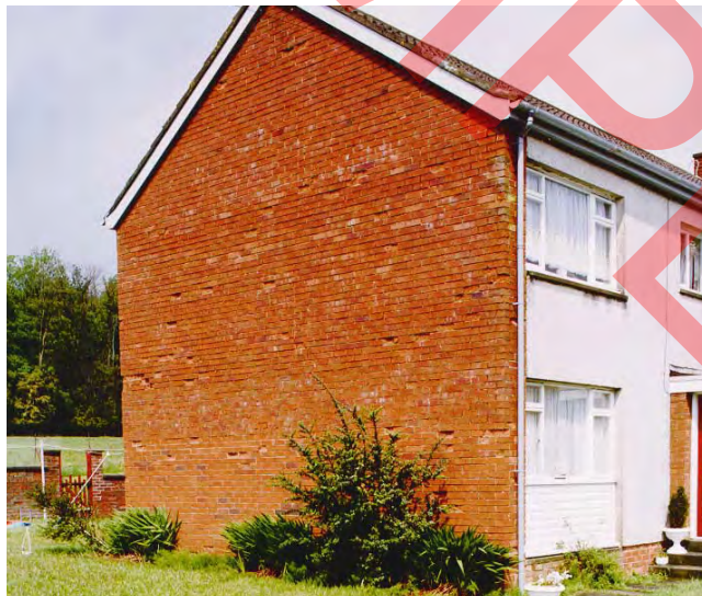
Frost damage to clay brick wall about 25 years old
