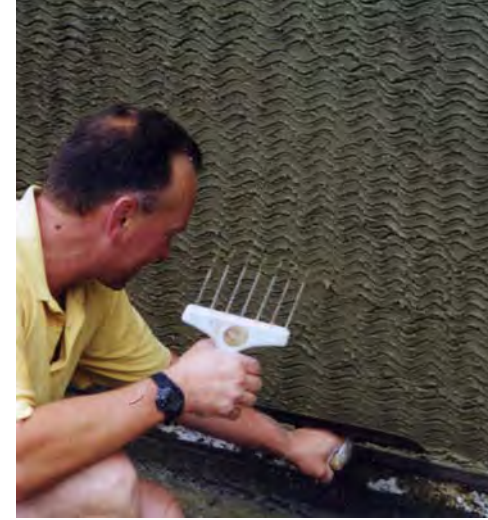
Figure 1 The scratch coat has been completed, and the detritus is being cleaned off the batten
