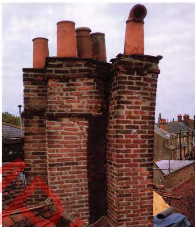
A common problem with chimneys - condensation leading to sulphate attack and causing twisting and leaning of stacks
