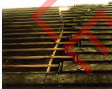
Inadequate bracing can lead to buckling of rafters across the whole roof.
